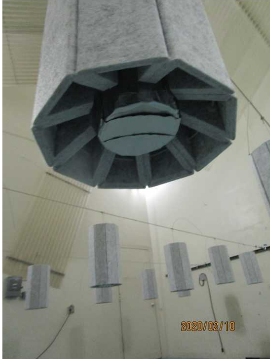
Figure 3 – Underside of individual fixture
